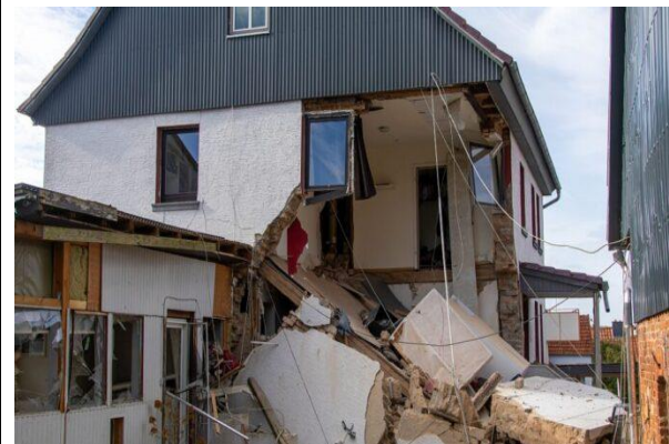
Figure 7: Explosion of a home storage tank leads to partial collapse (Vogelsberger Zeitung 2023)
