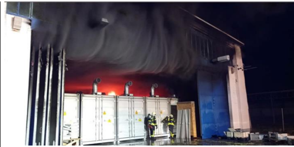
Figure 5: Fire at a large storage facility (KFV Märkisch-Oderland e.V. 2021)
