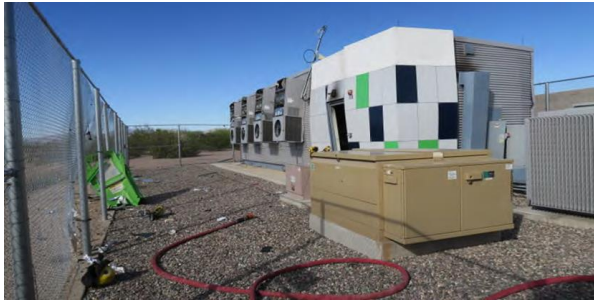
Figure 4: Explosion in large storage facility (Fire Safety Research Institute 2020)
